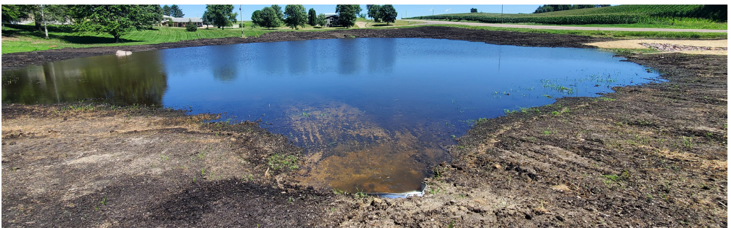
Contractors in summer 2020 excavated more of the wetland to increase flood storage, and installed a culvert connecting it to the upper watershed. Photo Credit: Le Sueur County SWCD
