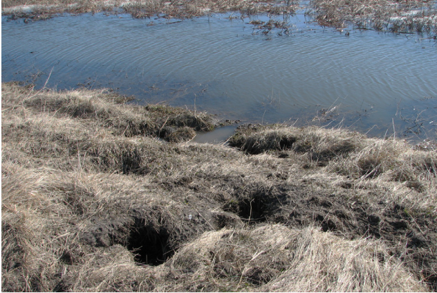
Figure 6.30 Muskrat burrows requiring an embankment repair
