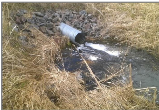
Figure 1. Upstream Drainage Tile Outletting into Restored Wetland
